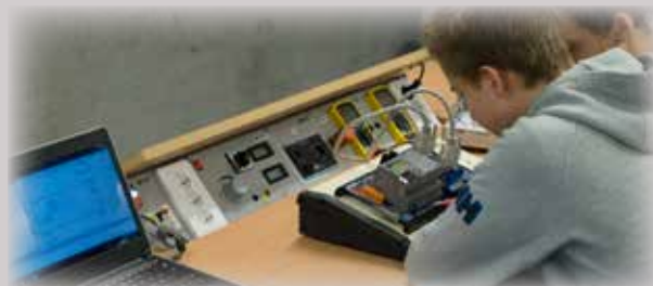
Power Distribution & Furniture for Lab
